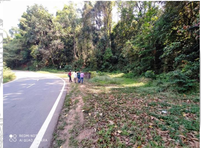
(j) Area along NH275 where subsidence of overburden material continuously occurs since 2013 in Koyanad Madikeri Kodagu
