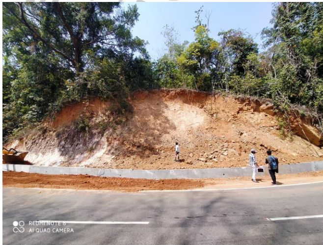
(i) Road cut slope along NH 275 near 10 th mile village Madikeri Kodagu
